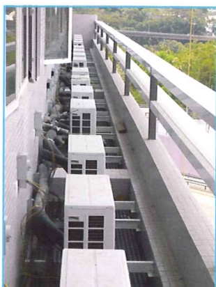
AC Condenser Unit Platform Sau Mau Ping ASD School Project
